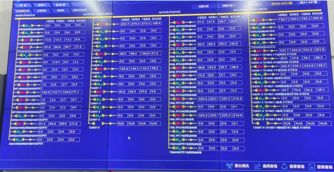
Energy Monitoring System (Example: Qinzhou Yard)
